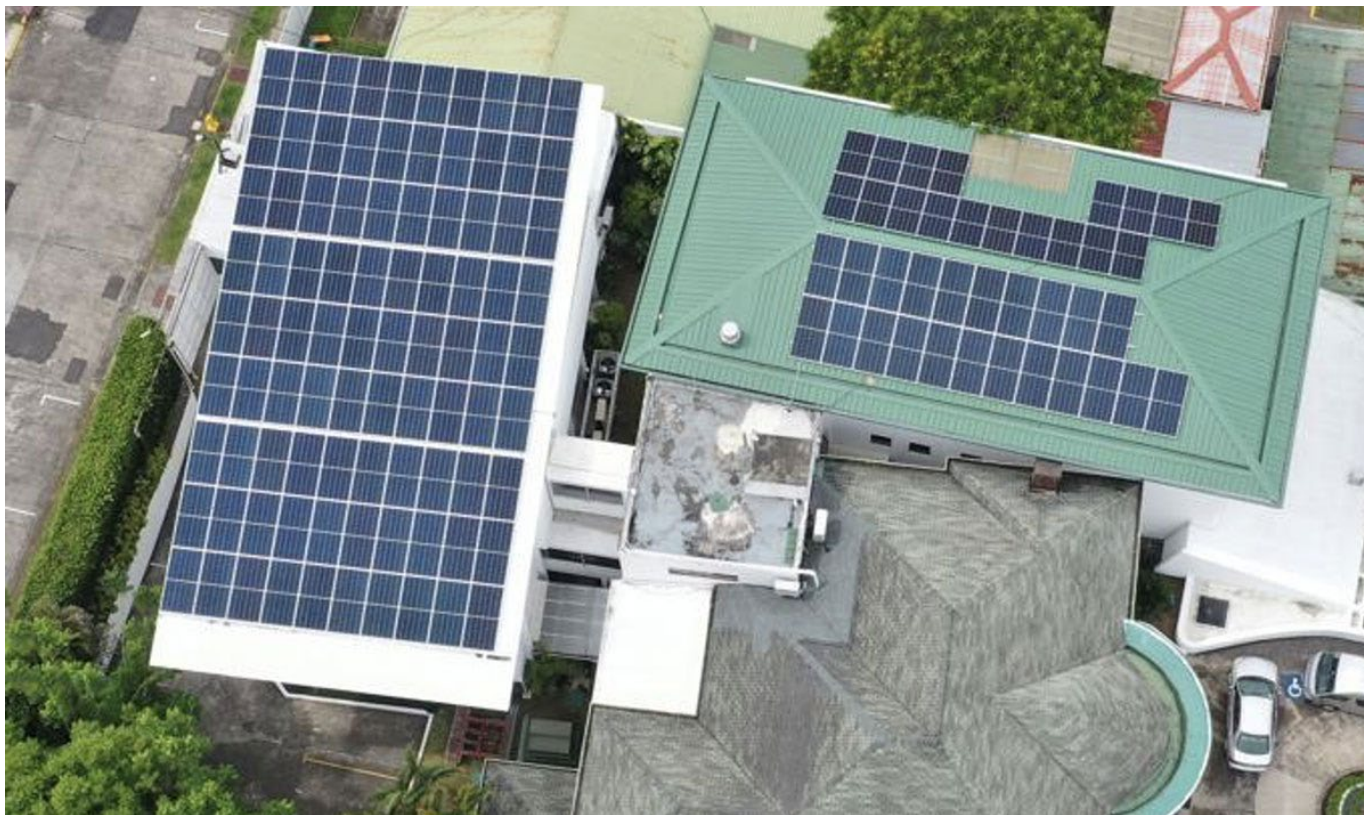
Aerial view of the solar panels installed on the premises of the Court.
